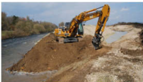
Figure 51. Restoration of the Danube. Work in progress between Hundersingen-Binzwangen (photo by Schnellbacher-Bühler A.)
